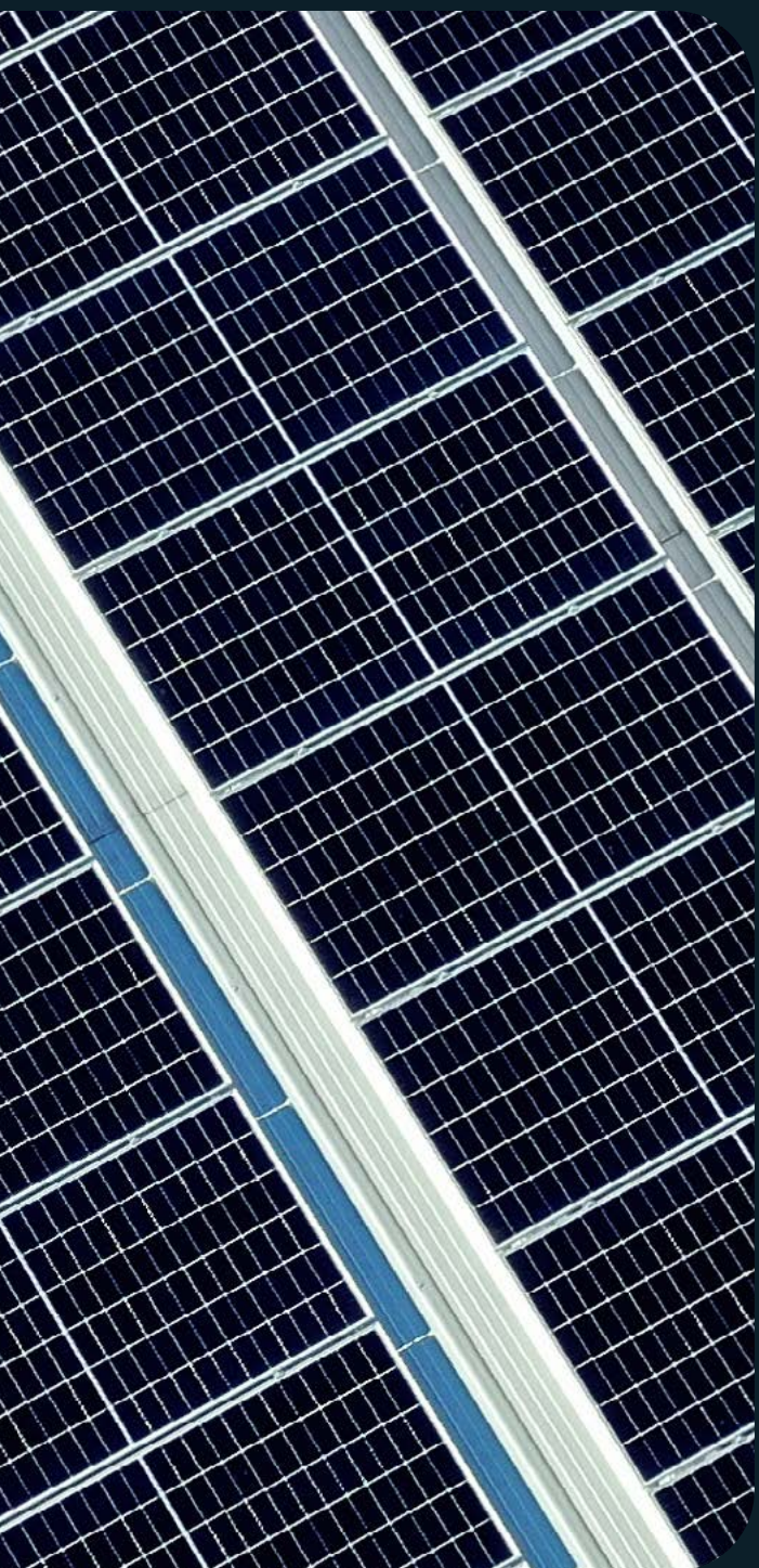
Solar PV panels
