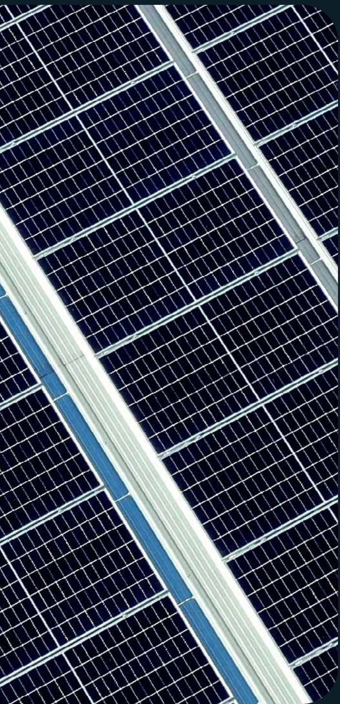
Solar PV panels
