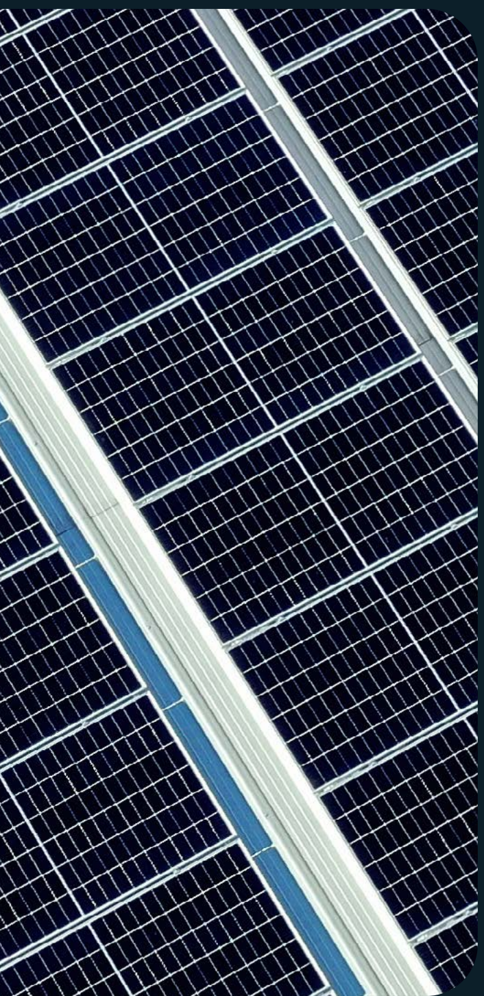
Solar PV panels
